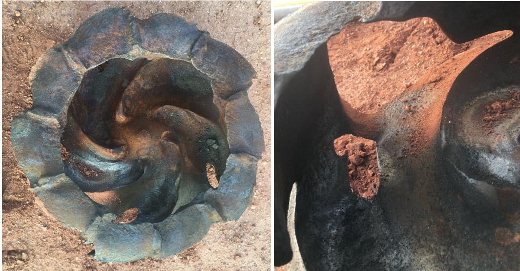
Figure 7. Two views of the worn impeller that was no longer able to maintain the required flow.
