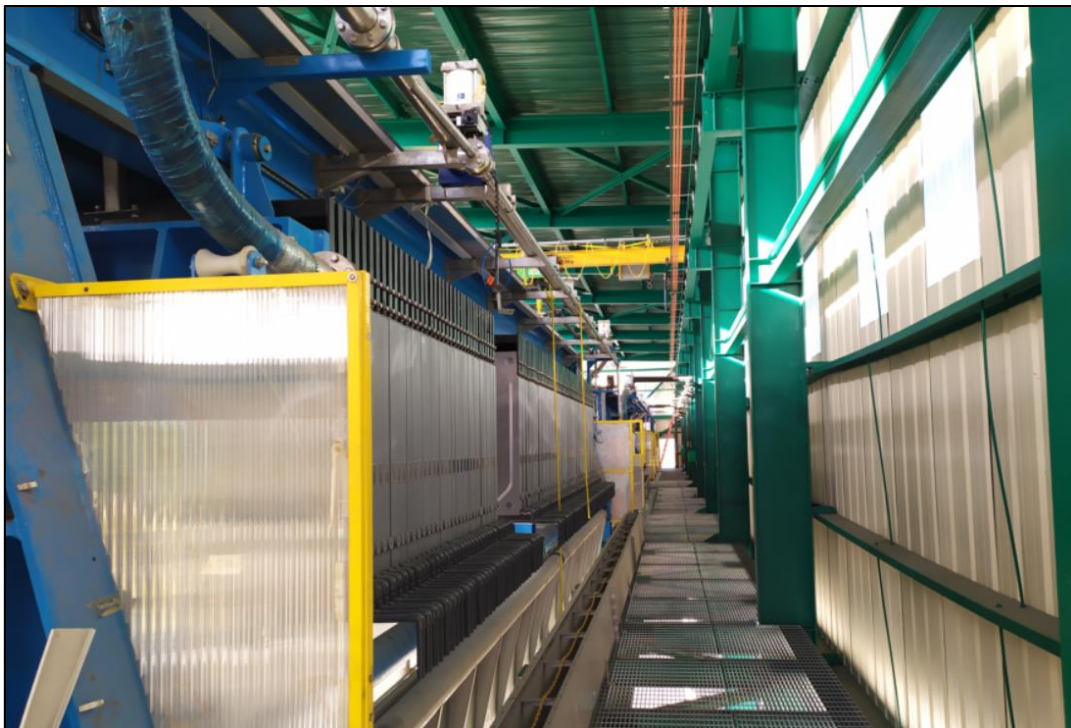
Figure 5 Filter presses installation for copper tailings treatment.
