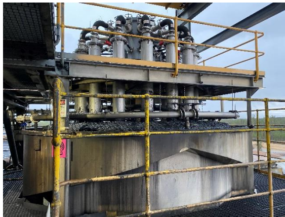
Figure 5 – Fully installed and operating Concorde Cell in the metallurgical coal washing plant
