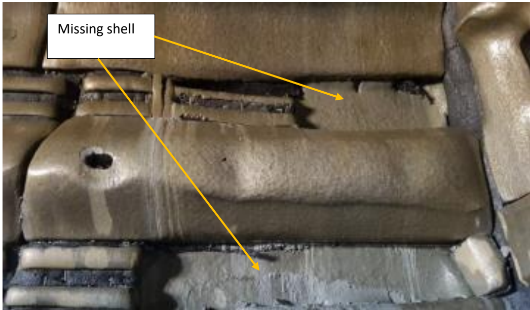
Figure 11: Hybrid steel liner failure
