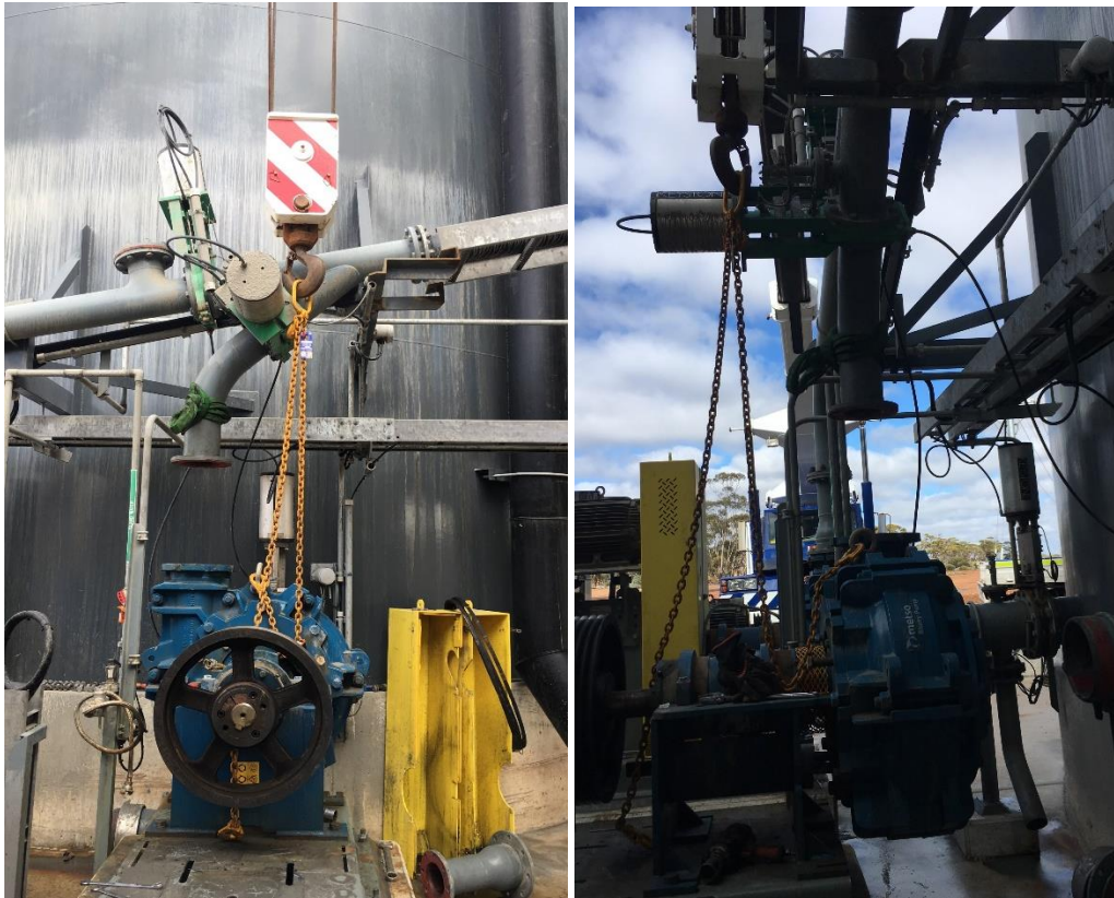
Figure 3. Actuator above pump centre-line Figure 4. Overhead pipework prevents vertical lift.
