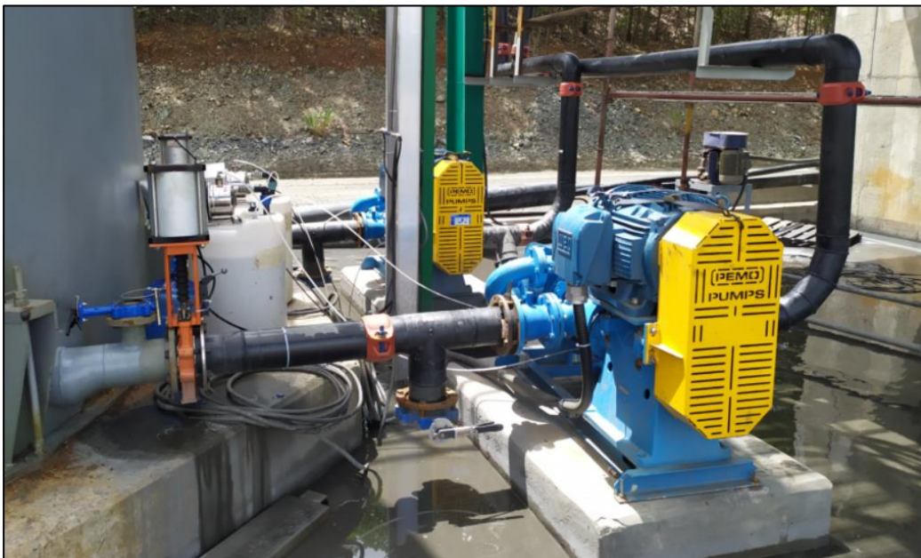
Figure 8 Slurry feeding pumps and flushing systems.
