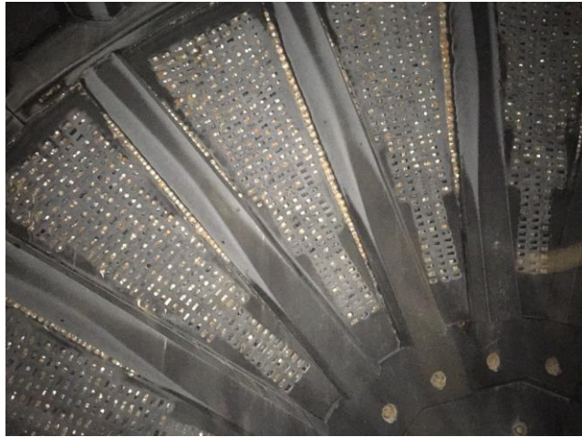
Figure 6: Original OEM supplied grates after 12-months operation (80% pegging in some areas)
