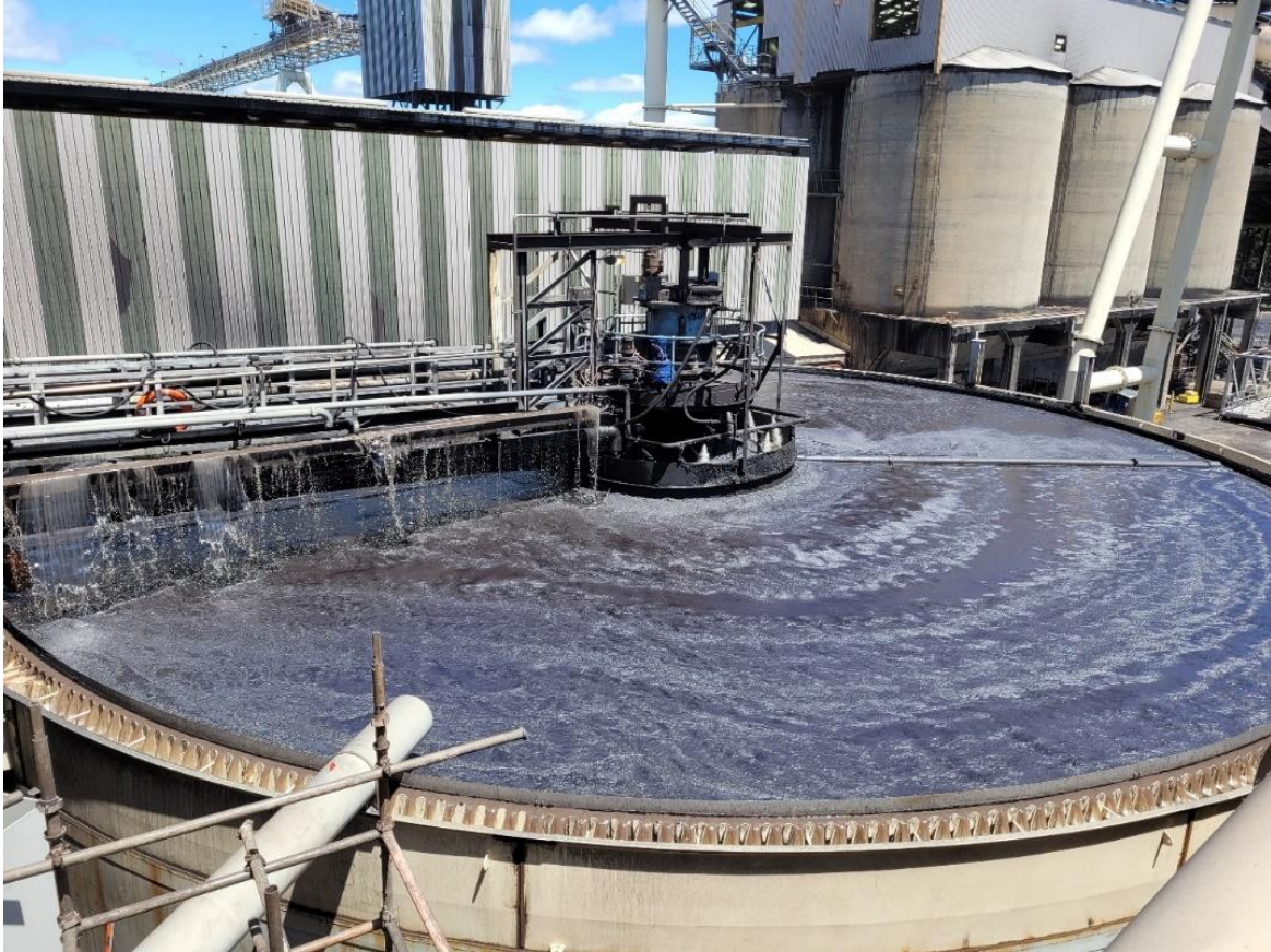
Figure 4: Existing Coal Thickener Before Upgrade of bridge and froth management, note the waterfall style froth suppression curtain on the left-hand side of the centre well and rotating froth boom
