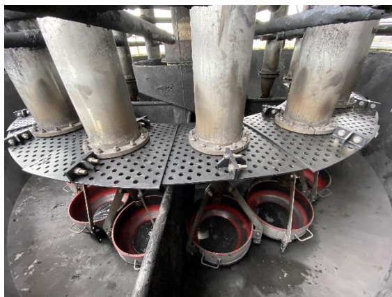
Figure 6 – Concorde Blast Tubes and impingement bowls inside the existing SAP flotation tank
