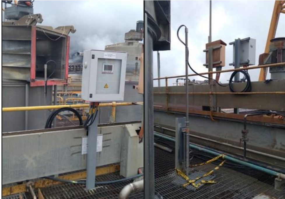
Figure 1: C2 Meters control panel, and probe installation
