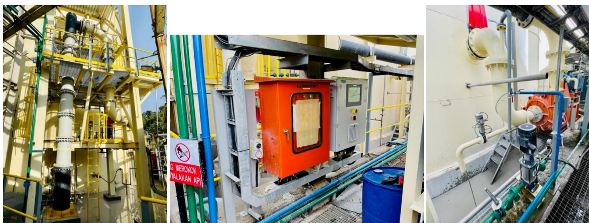
Figure 8a, 8b & 8c – Images of some portions of the high shear leach reactor installation at PT IMK
