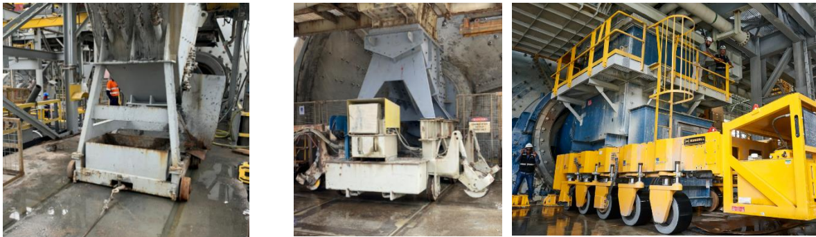
Figure 4 – Examples of different feed chute removal methods. Left: Winch with one-directional rail base. Middle: Powered two-directional rail base. Right: Rubber-tyred transporter
