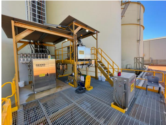
Figure 11 - OLGA and CS installation at the Gruyere Mine
